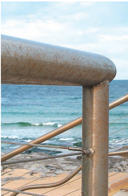
Tea staining of stainless steel in a coastal environment shortly after installation.
