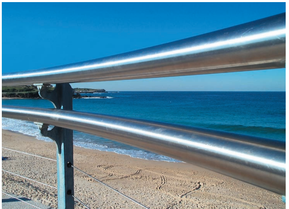
Successful use of stainless steel after more than 14 years service in a coastal environment.
